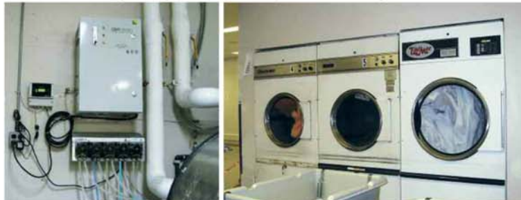
Top: Roger Parker (L) and John Madill (R) with UniMac washers. Below: Left: The ozone-generating system. Right: The dryers, newest one at right.
